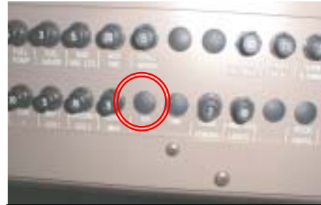
Figure 2-6 Circuit breaker location (Typical)
